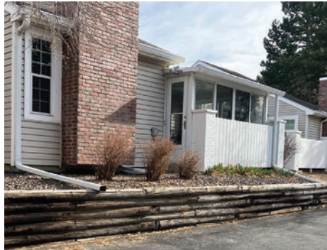
Deteriorated Wooden retaining wall in CP-3
